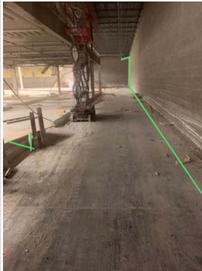
Storm Drainage- Following the Eastern foundation wall, draining South.
