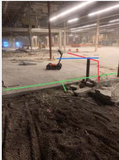
(Abandoned) Electrical & Refrigerant lines
